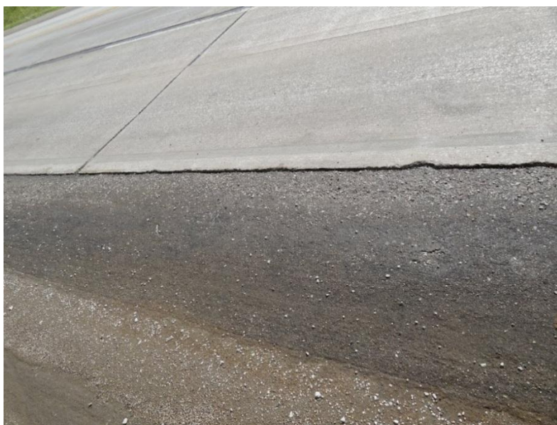
Figure 20. Southbound shoulder of US 169 south of Algona
