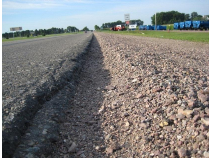
Figure 1. Edge rutting on granular shoulders (by Thang Phan)
